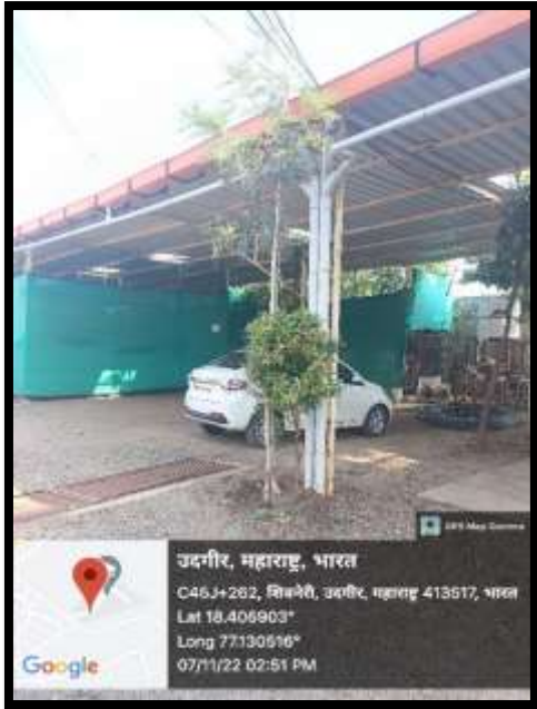
Rain Water Conduction PVC Pipes
